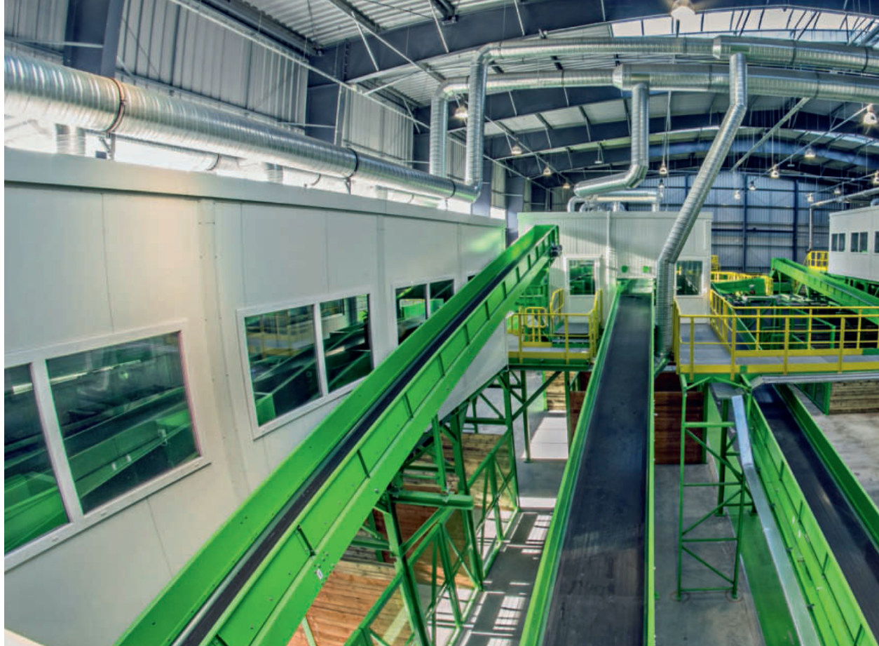
6 ▶ View of the plant for waste sorting at the new MBWT plant in Żary/Poland
